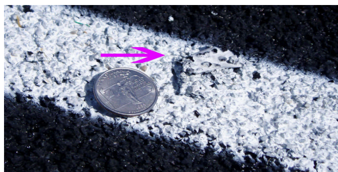
Excess resilient material on surface (has since been corrected)
