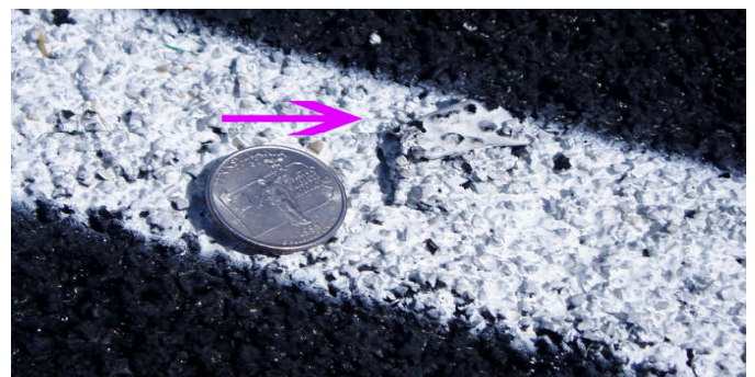
Excess resilient material on surface (has since been corrected)
