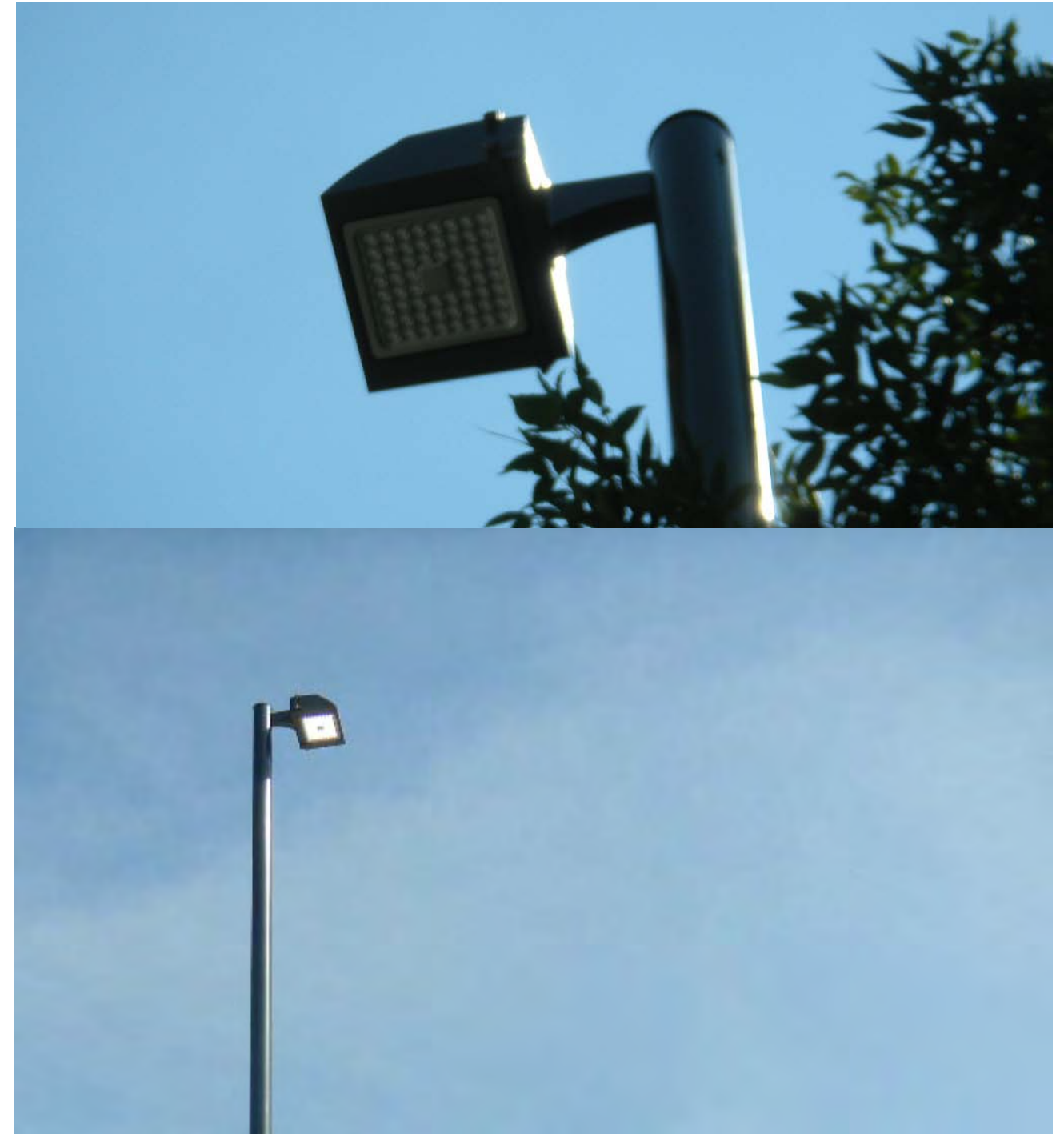
LED Site Lighting Fixtures Installed at Cather in 2012
